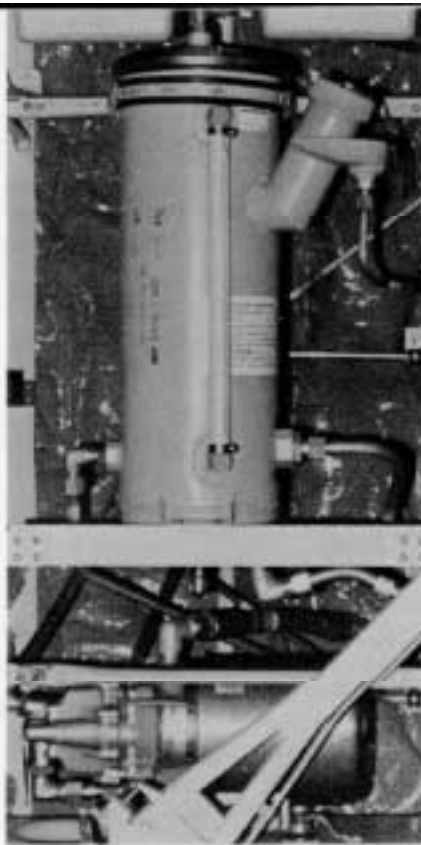
Auxiliary hydraulic system reservoir and pump.
