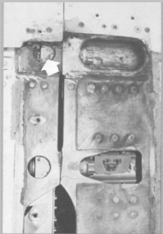
Entrapped moisture caused corrosion in this rainbow fitting.
