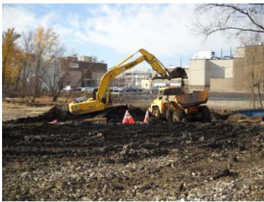
1. Loading of soils for disposal at licensed landfill sites. More than 31,000 tons have been removed.
