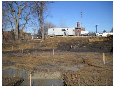
2. View of completed northwest excavation area in the northern portion of the site.
