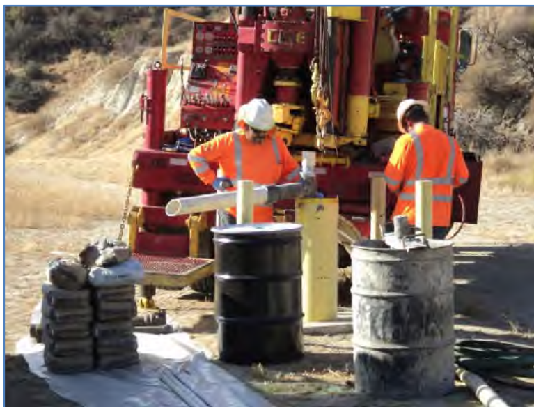
Photo No. 2: Close up of wellhead prior to placing grout. Horizontal pipe is used to divert displaced groundwater into a 55-gallon drum.
