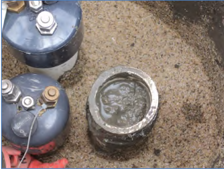
Photo No. 3: Close up of the TT-MW2-38C well casing after well destruction.
