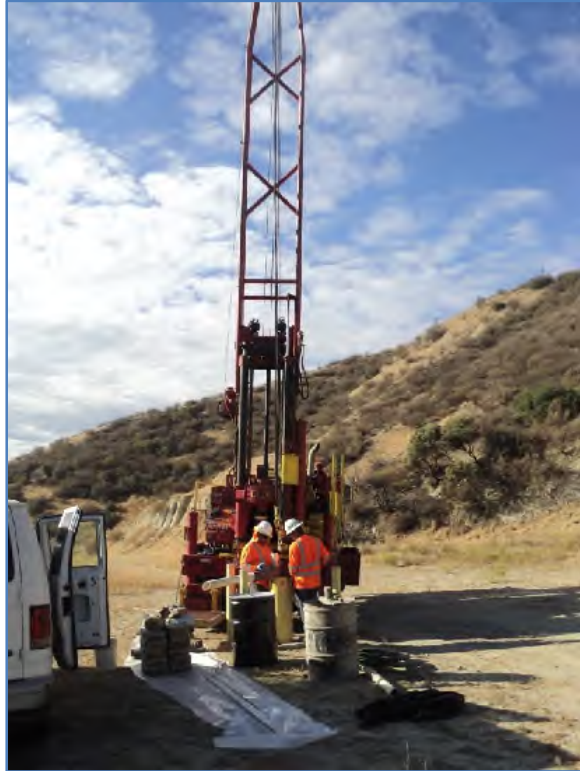
Photo No. 1: Drill rig set up on TT-MW2-38C in preparation for well destruction.
