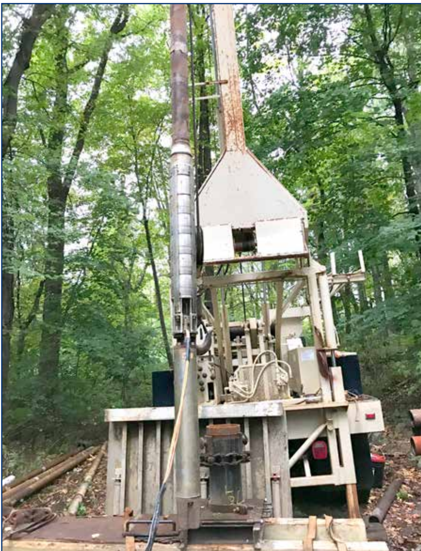
A down-hole rig is used to access the existing remedial diffusion well for maintenance and cleanout.
