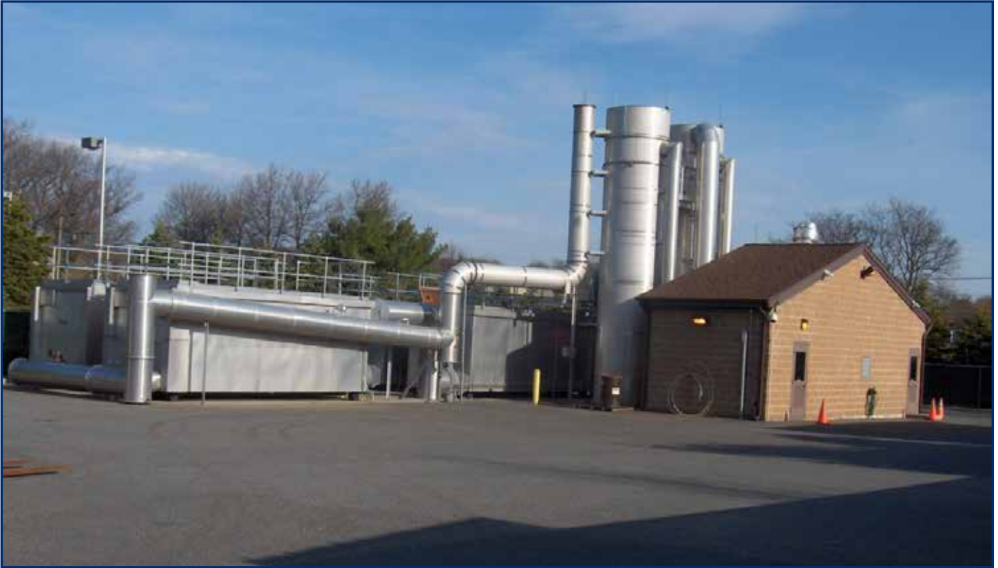
On-Site (OUI) Groundwater Treatment System
