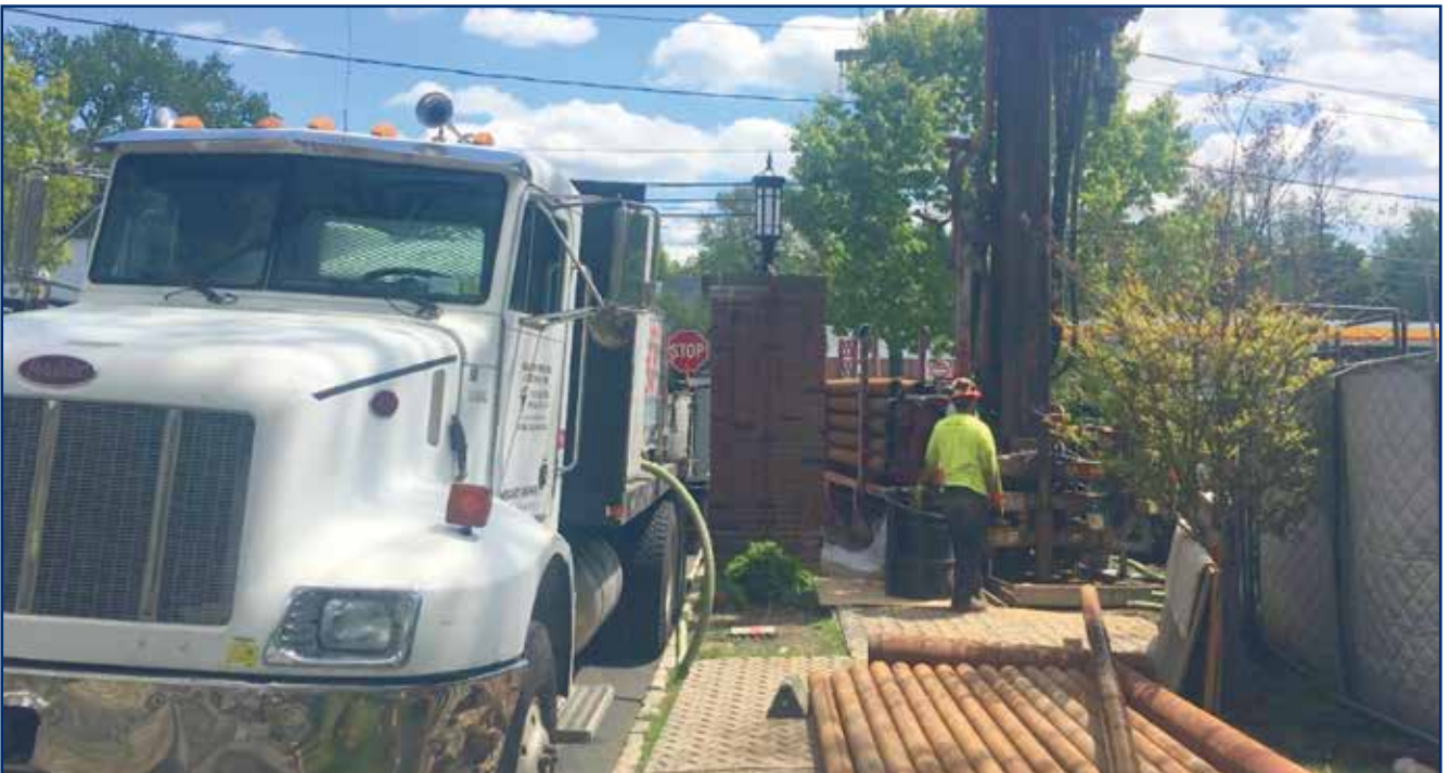
A similar well was installed in 2019 in the Village of Russell Gardens.
