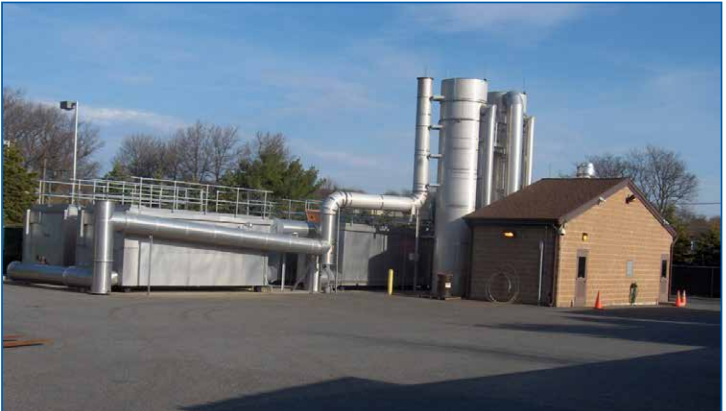
On-Site (OU-1) Groundwater Treatment System
