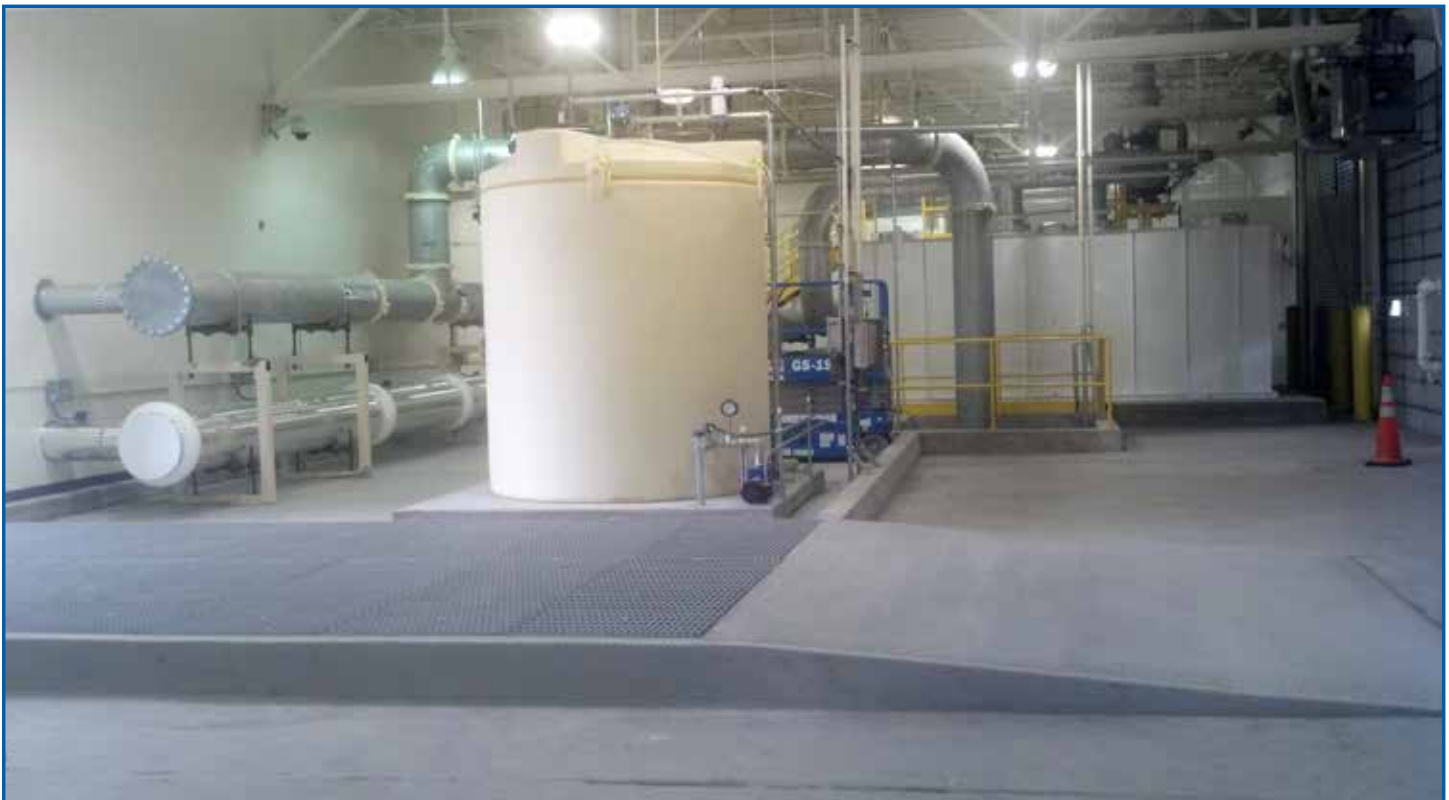
The sub-slab depressurization system (SSDS) ensures safe air quality inside the main building
