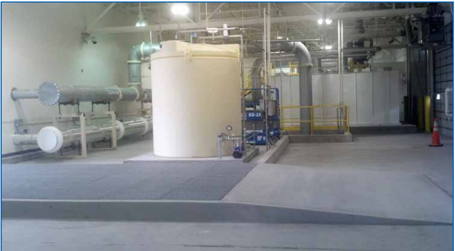
The sub-slab depressurization system (SSDS) ensures safe air quality inside the main building
