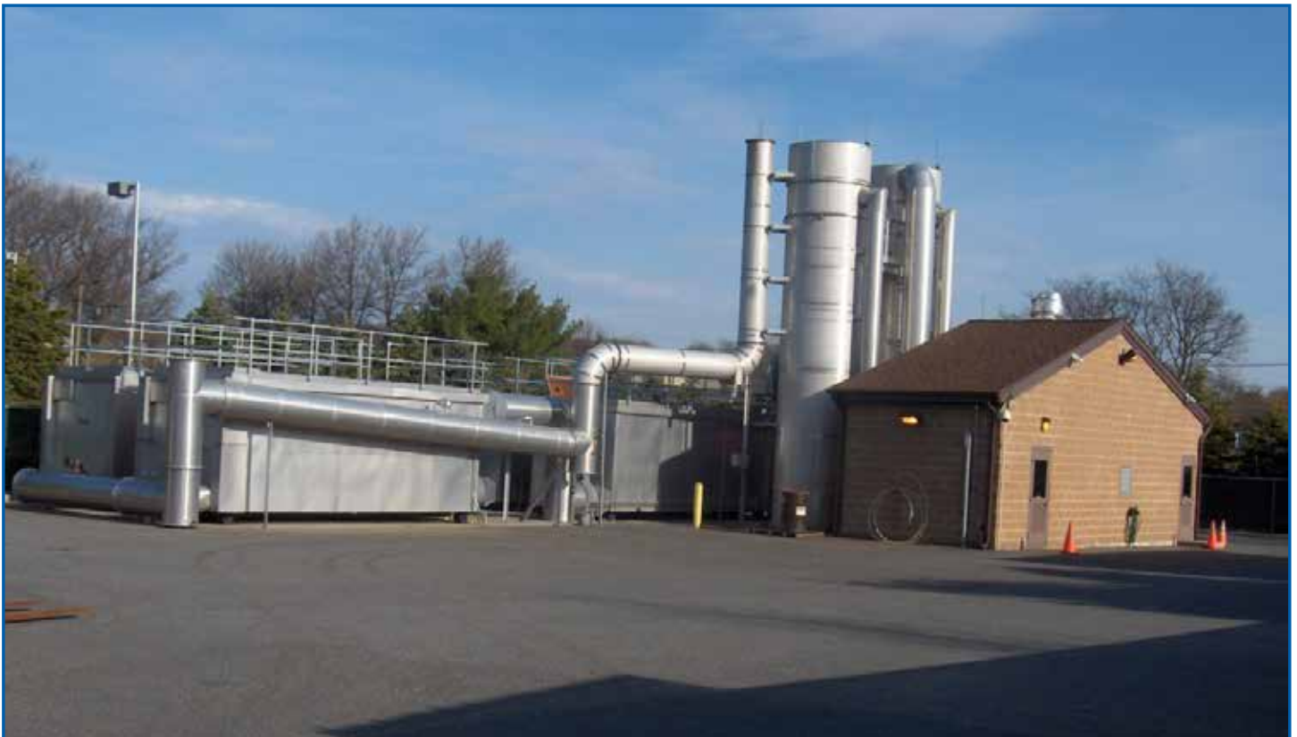
On-Site (OU-1) Groundwater Treatment System
