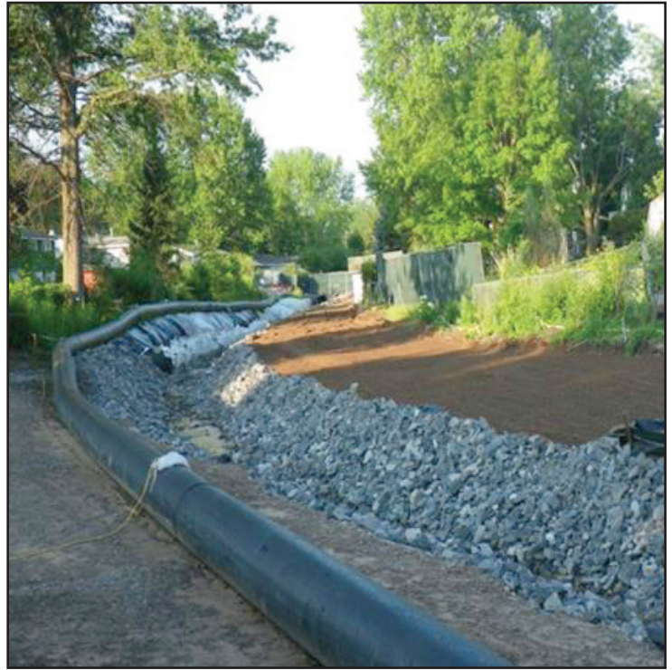
Continuing remediation and restoration of former gabion-lined portion of brook near Brookview Lane.
