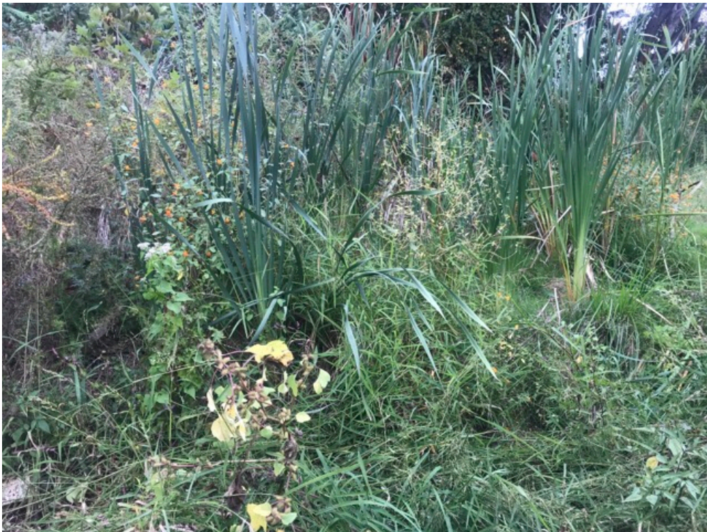
Figure A-73. Soil eroding from under the matting on the right bank at Station 01+67, 2018 (top) and 2019 (bottom).
