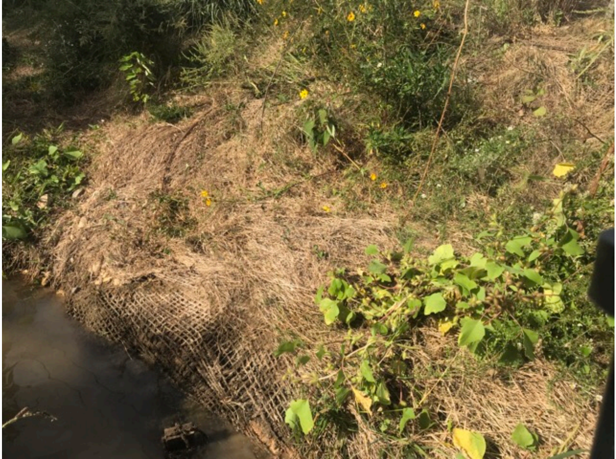
Figure A-7. Left streambank at Station 01+57.
