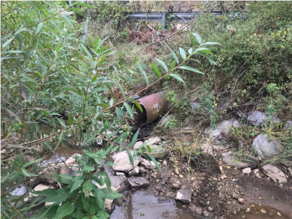
Figure A-74. Outfall and guard rail on the right bank at Station 01+99, 2018 (top) and 2019 (bottom).
