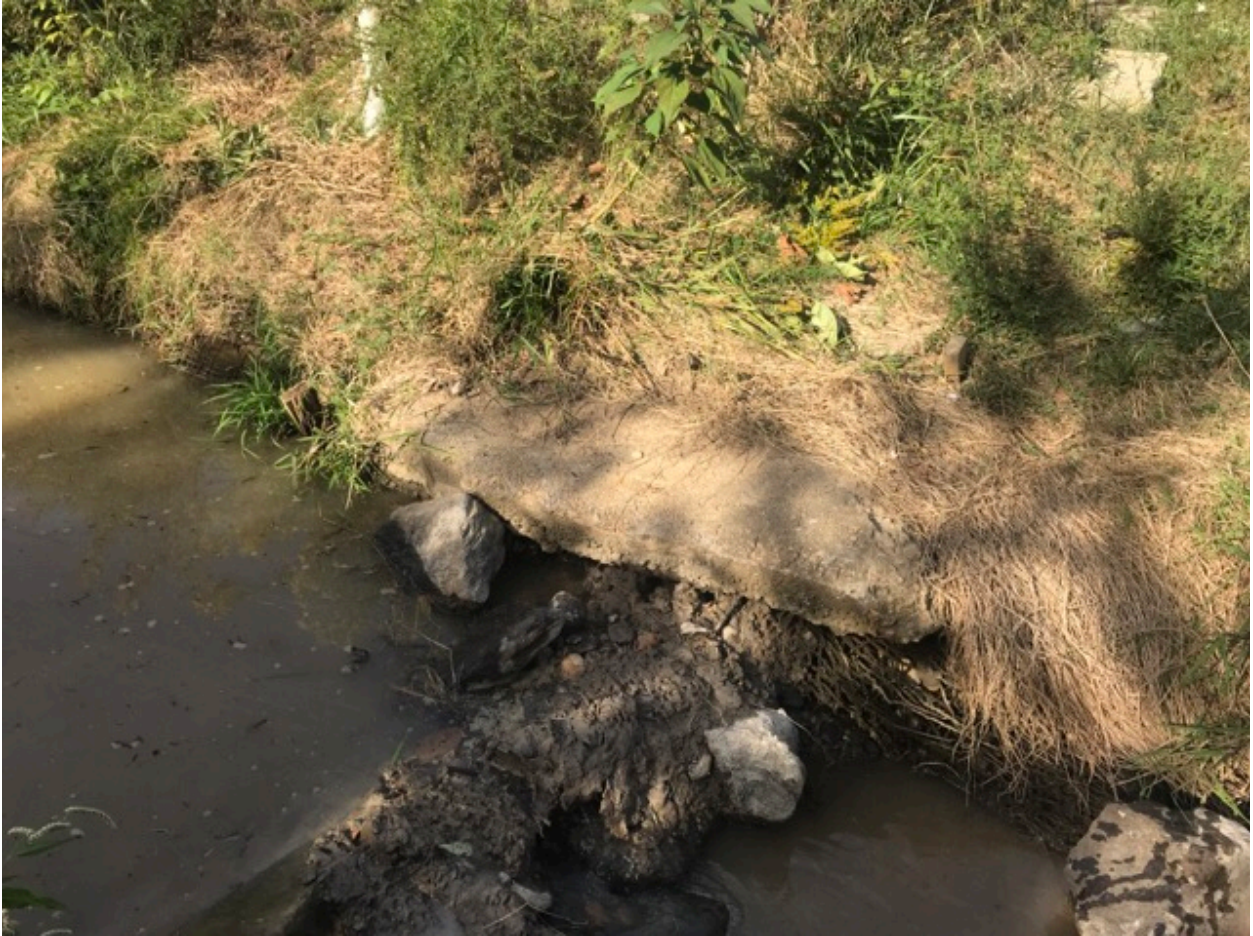
Figure A-11. Left streambank at Station 01+98.
