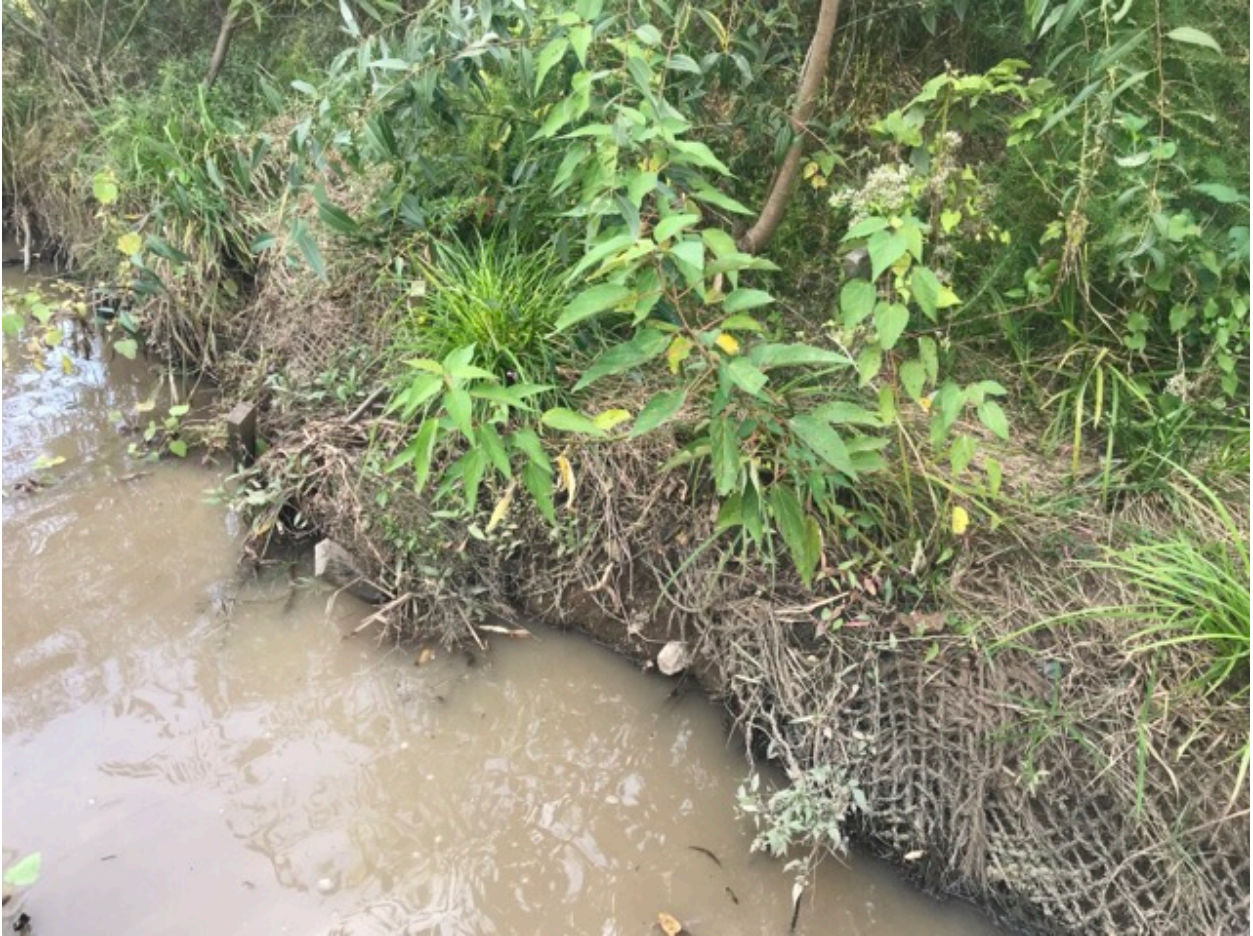
Figure A-13. Left streambank at Station 02+32.
