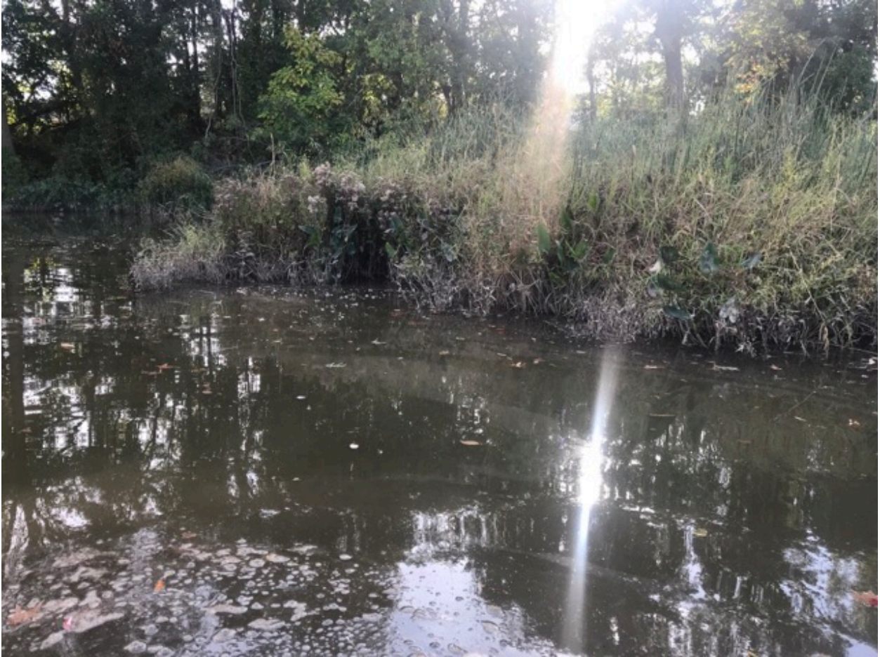
Figure A-27. Left streambank, in backwater area at Station 07+57.
