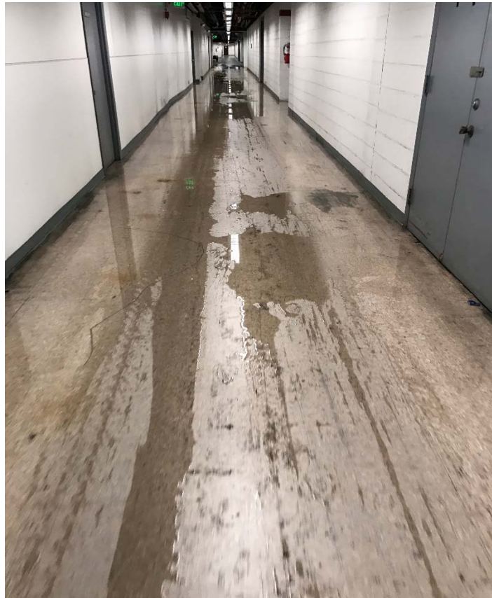
Flooding down hallway in northern portion of Building C basement
