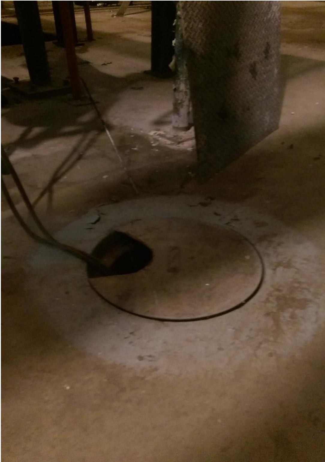
Photo 3 – Sump pit near column D24 with 170 ppb detection for trichloroethene using the Frog 4000™.
