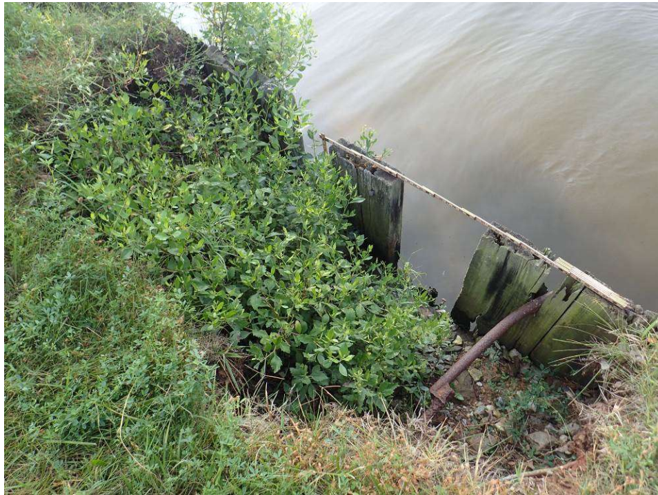
Photograph 21. Backfill loss and vegetation behind broken breastwall timbers.
