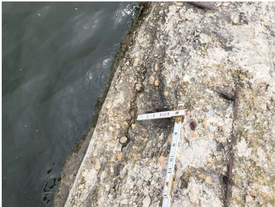
Photograph 14. Typical deterioration of concrete deck, showing spalling and exposed reinforcement.
