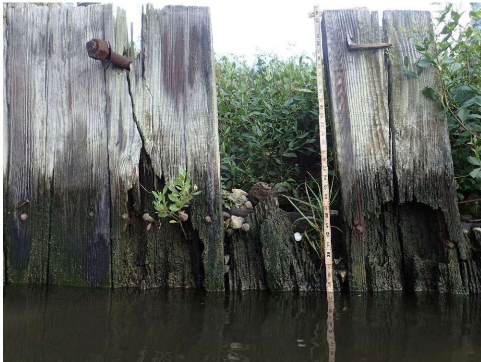
Photograph 20. Broken vertical timbers at waterline with associated fill loss.
