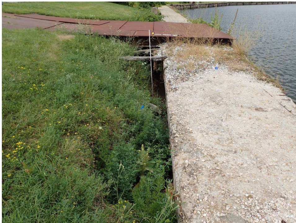
Photograph 12. Section “H”, typical embankment erosion behind seawall.
