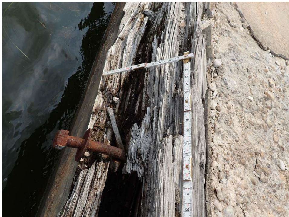
Photograph 16. Severe deterioration of timber fender at edge of concrete deck.
