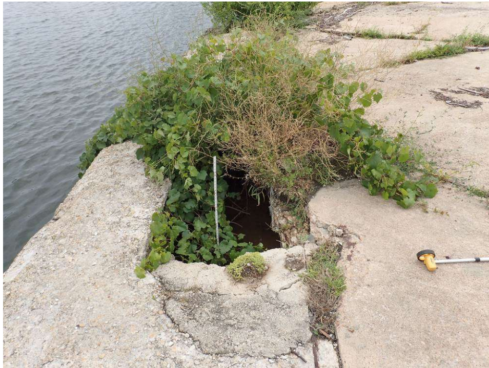
Photograph 15. Section “H”, failed area of concrete deck with backfill loss and vegetation growth.
