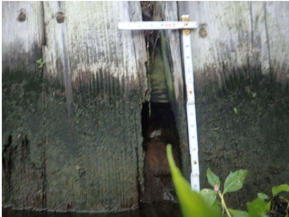
Photograph 19. Decay and 100% section loss of breastwall timbers in tidal zone.
