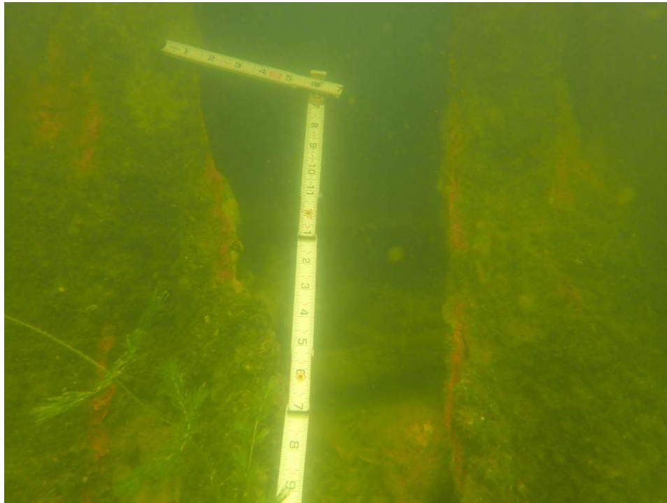
Photograph 9. Typical severe deterioration of steel sheet piling.
