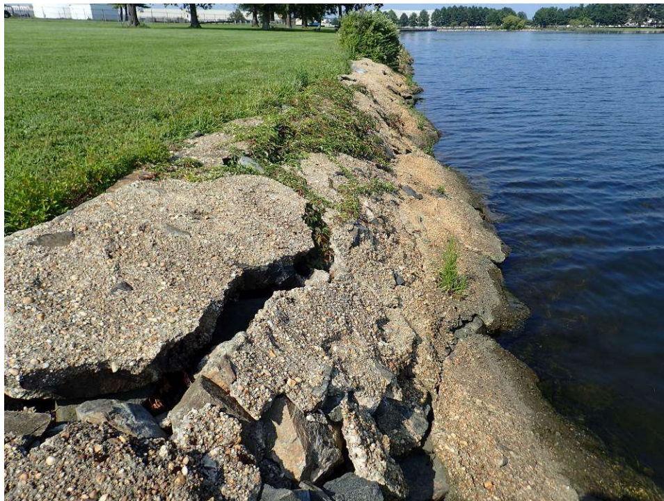
Photograph 18. Longitudinal cracking in upper concrete of stabilized riprap slope.
