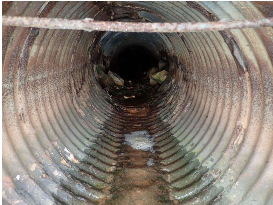
Photograph 17. Outfall pipe with areas of 100% section loss.
