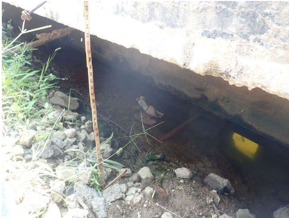
Photograph 13. Typical fill loss beneath concrete deck, showing area of 100% section loss in steel sheet pile at lower right.
