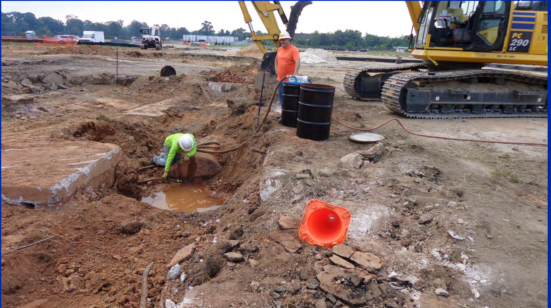
The first unexpected underground storage tank held waste water and had stored petroleum/diesel. Contents were drained, drummed and tested for proper disposal.
