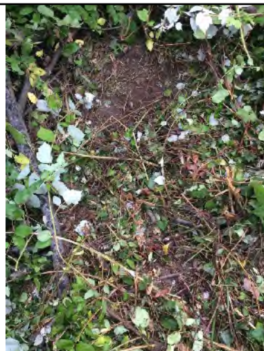
Surface vertical pipe dug down 1' and broken up with sledgehammer so that no pipe is visible from surface.
