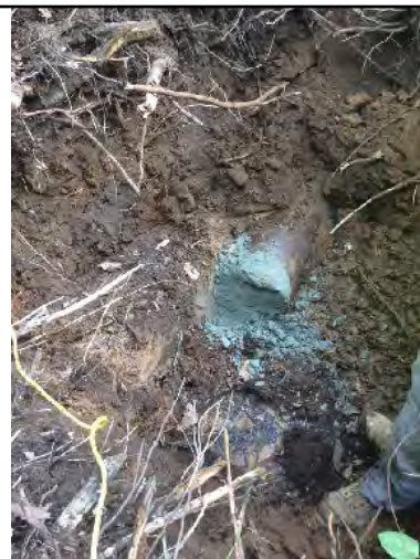
Pipe was broken, bank side removed, land side filled and sealed with concrete.
