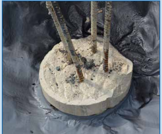
Vapor barrier components are sealed around all penetrations, such as this foundation pile.
