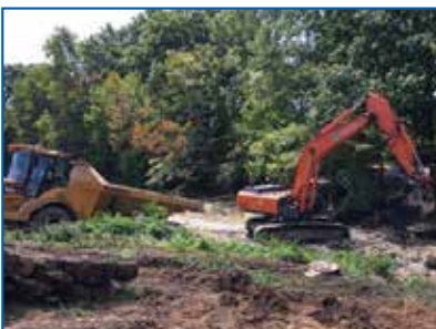
Excavators in the creek removed contaminated sediments to transfer by trucks for removal.
