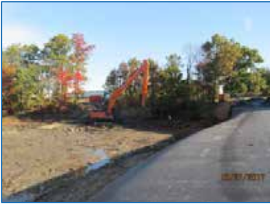
Dams built in Cow Pen Creek created dry excavation areas. A rubber water-filled bladder dam was constructed in the lowest excavation section where the creek was deepest and widest.
