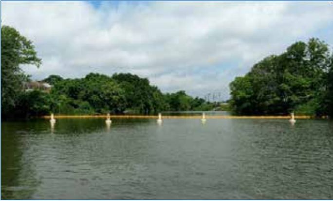
Lighted buoys and a silt curtain were installed at the mouth of Cow Pen Creek to prevent boaters from entering and silt from leaving the work area.
