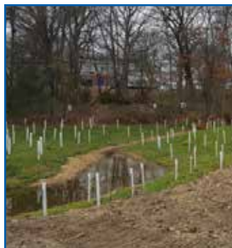
Following sediment excavation, the creek was restored to resemble the stream course before work began by rebuilding meandering curves and planting native vegetation.
