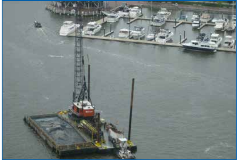
Barge with crane and clamshell bucket will be towed from Baltimore and will be located inside the boom line and silt curtains at the dredge site.
