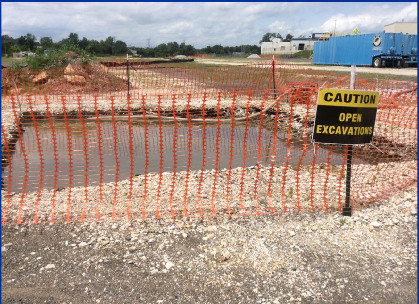
Storm water was pumped out and sent to storage tanks located in Block G.
