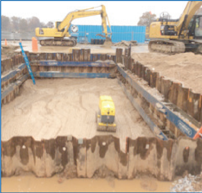
Shoring was needed to safely access underground storage tanks in Block F.
