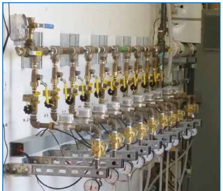
Equipment inside the trailer distributes lactate (sugars) and water through a system of underground injection wells to activate bioremediation.
