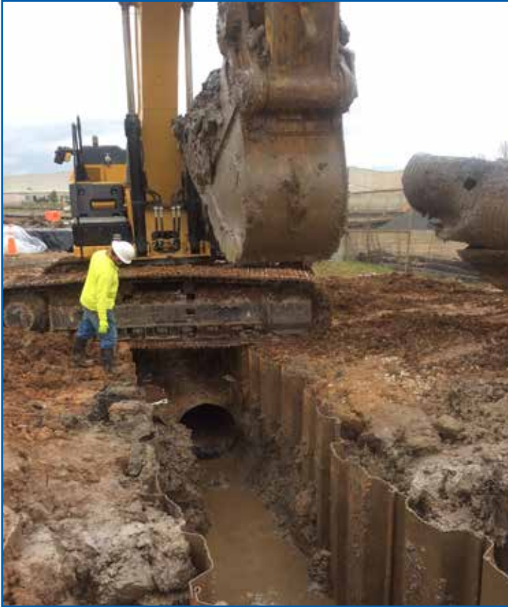
A storm drain outfall required repair in the bulkhead at the corner of Blocks D and D Panhandle.
