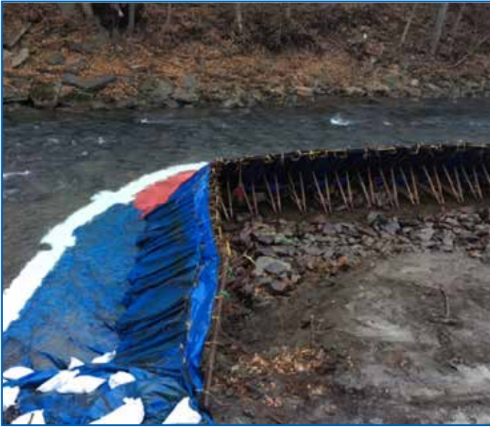
An example of a coffer dam which separates a stream from a dry work area.
