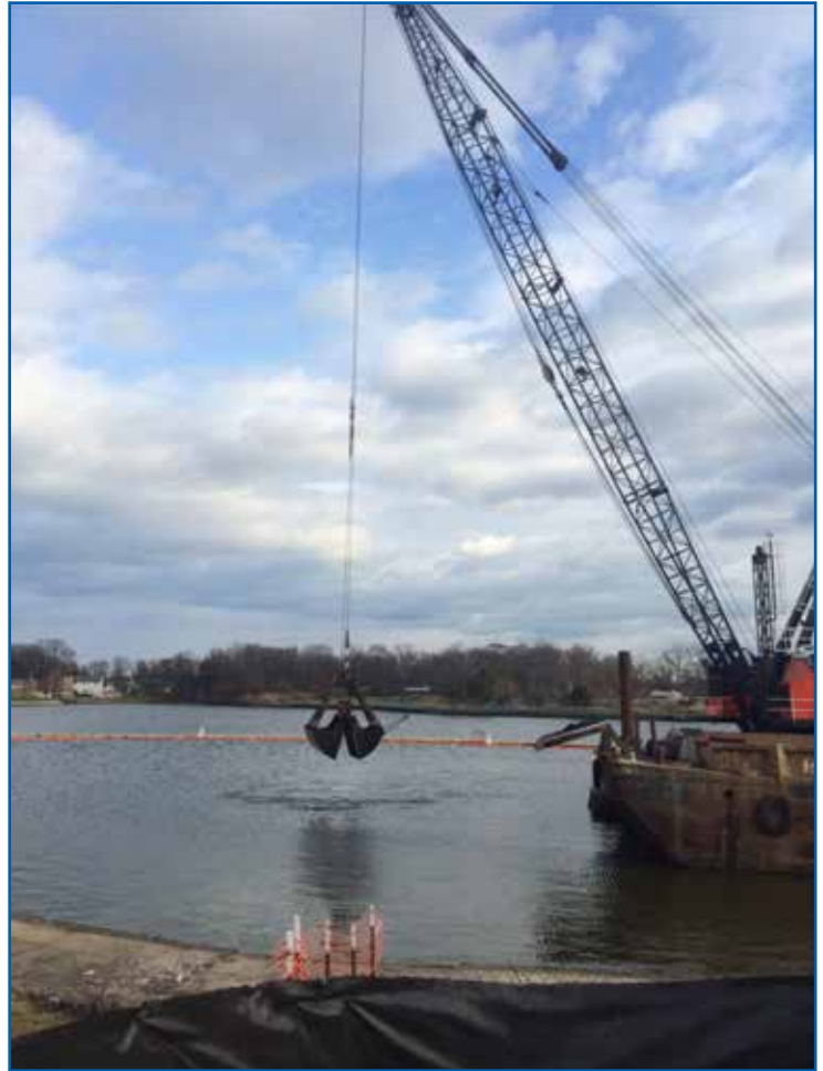
Dredging in 2014-2015 at Outfall 005 used an environmental “clam-shell” bucket to seal sediments before removing them.
