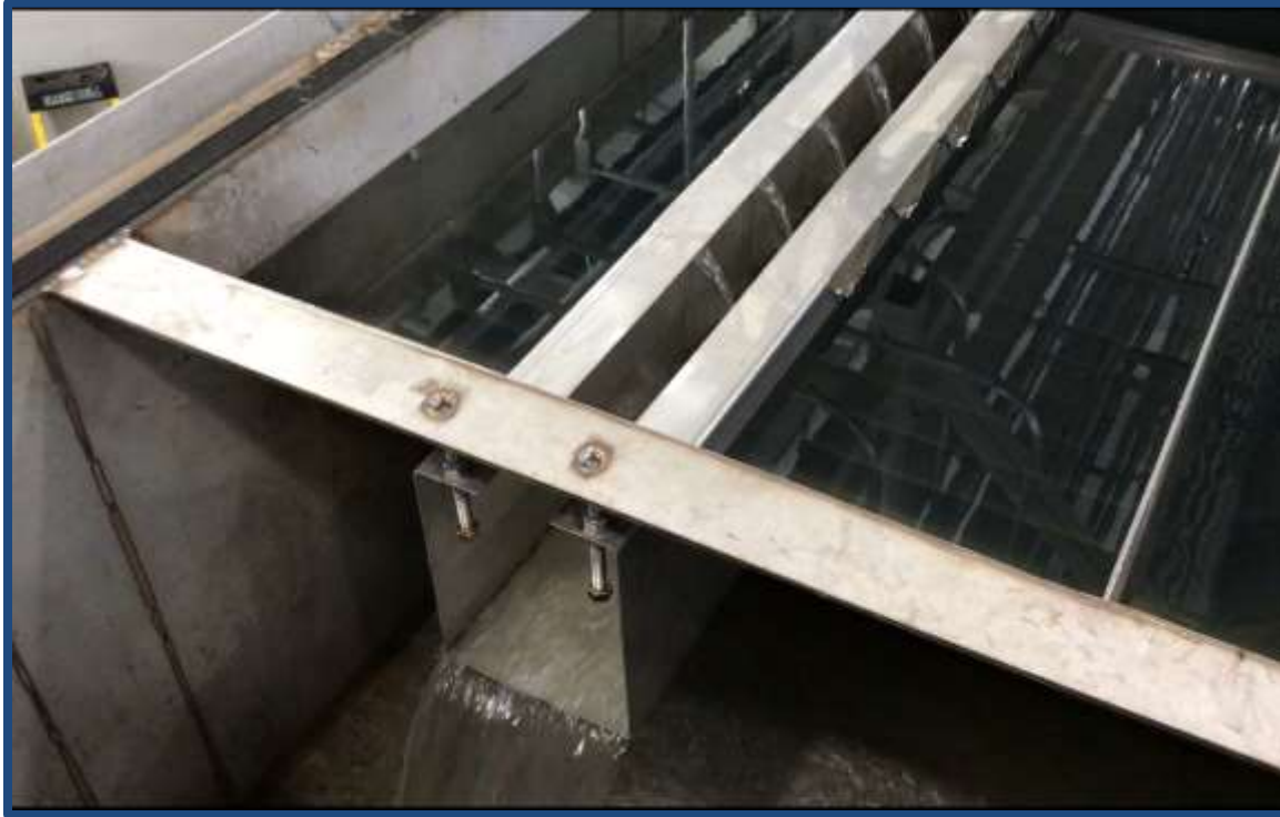
Clarifier clear water overflow
