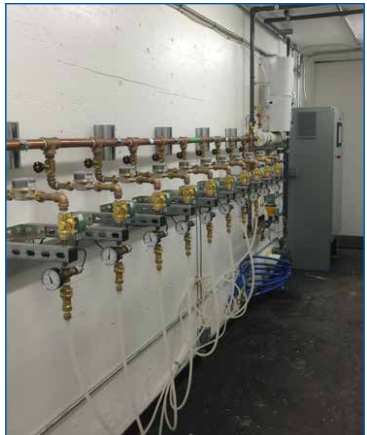
Groundwater injection ports.
