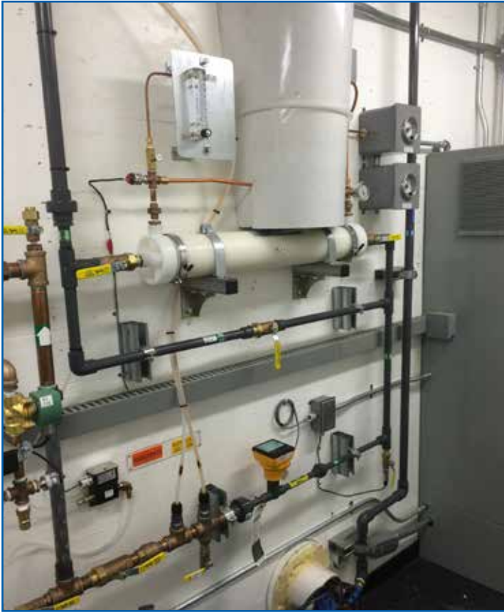
Groundwater injection system components.
