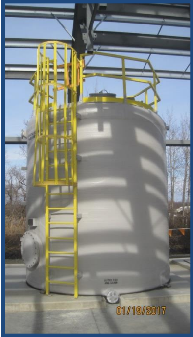
Dirty Back Wash Tank
