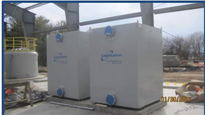
Decant Tank and Vapor Phase Granular Activated Carbon Units
