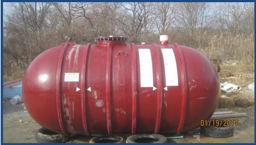
Sanitary Holding Tank
