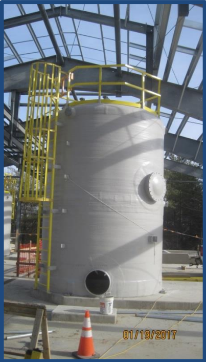
Sludge Holding Tank
