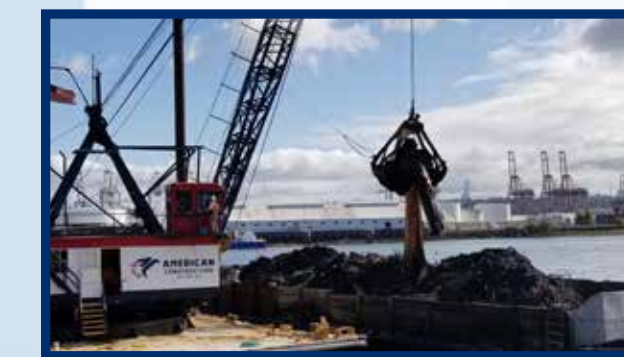
Decision Unit 5 Supplemental Dredge and Fill: March 9 – March 25
