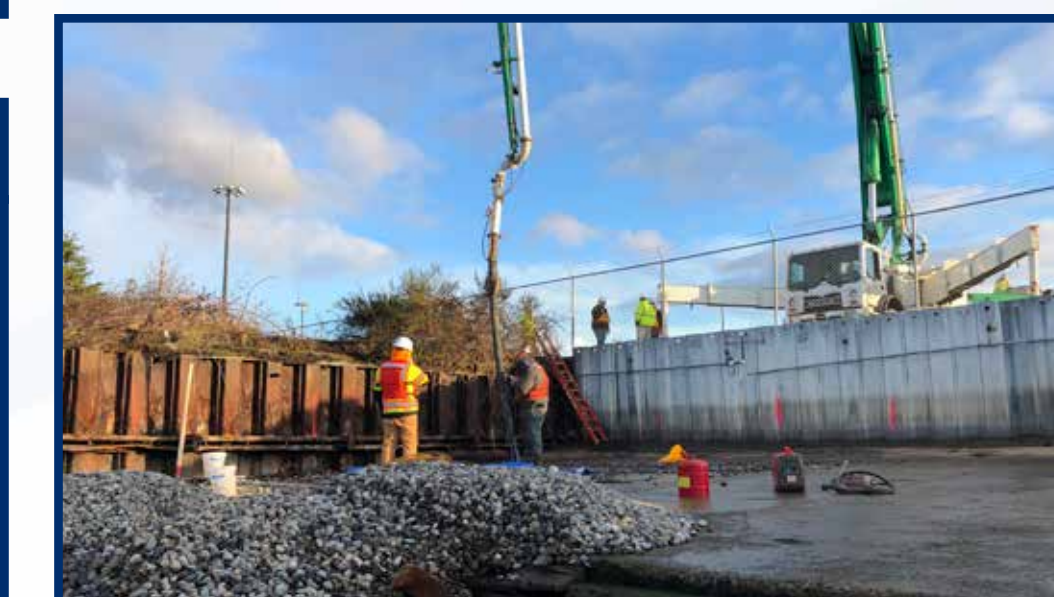
Grout was placed, to prevent undermining, under the existing concrete slab in the shipway to stabilize it.
