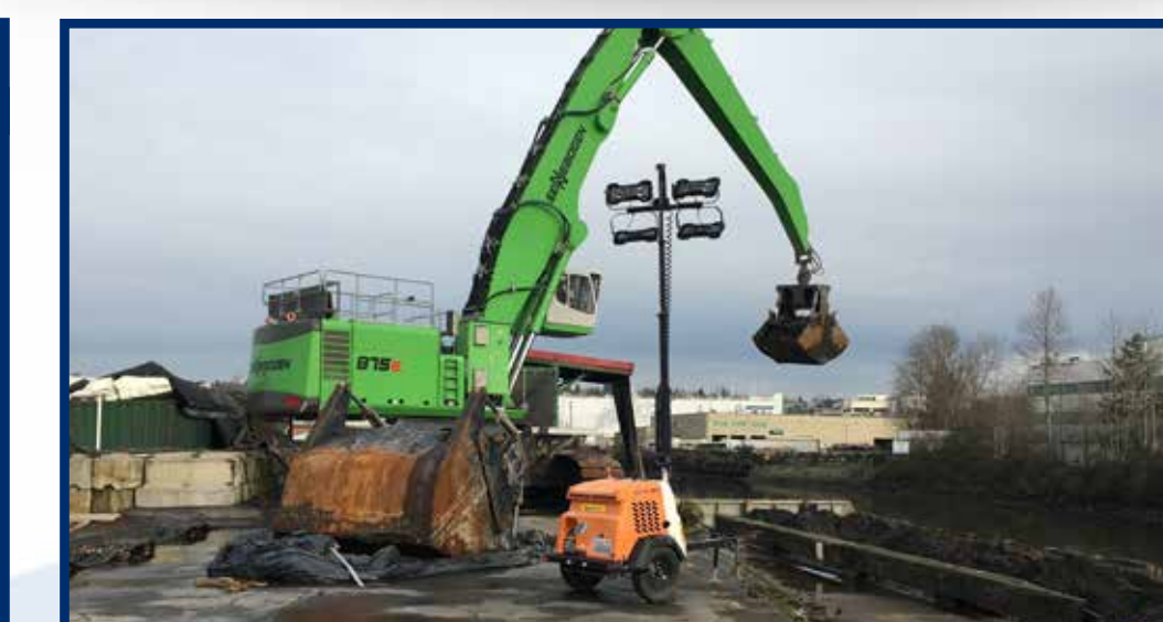
Excavator unloading dredged sediment from barge to sediment transloading facility where rail cars are loaded.
