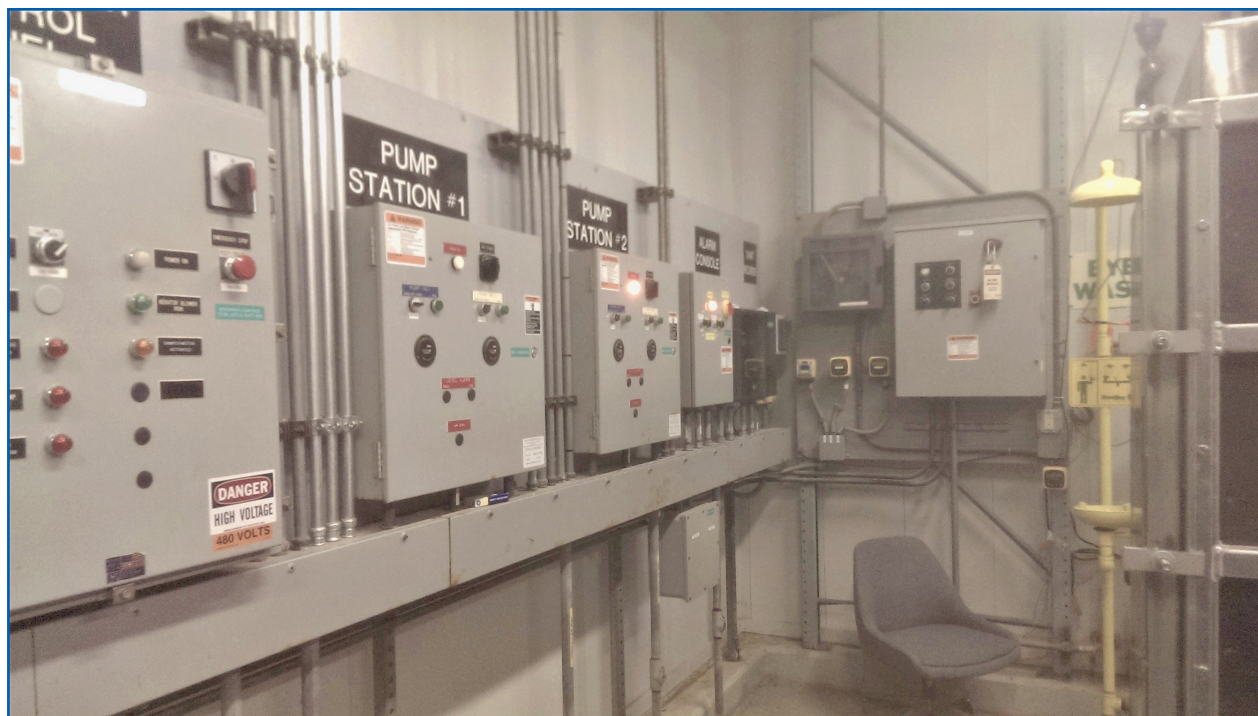
Pump Controls inside the Groundwater Collection and Treatment System (GCTS) Facility
