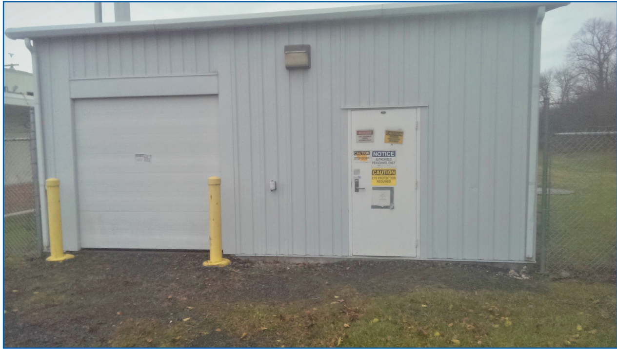
Groundwater Collection and Treatment System Facility
