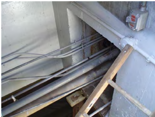
28.) Trench PUM Vent House Interior; Stoddard Odor
