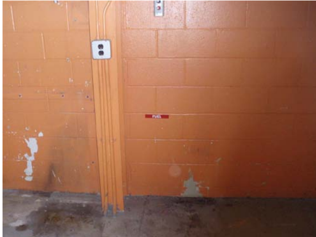
37.) Interior Rooms, Open Office C Trench
