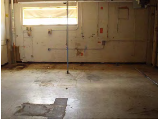
33.) Interior Rooms, Open Office C; Sanitary Drain
