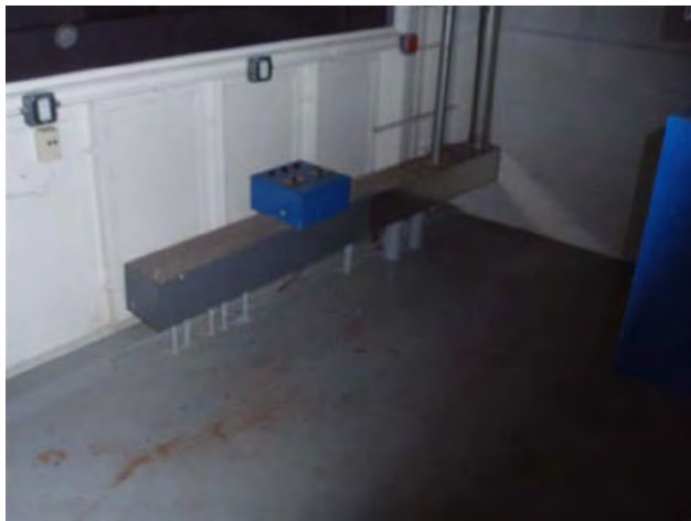
14.) Control Room, Elec. Entrance
