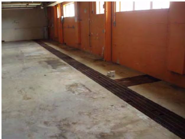
36.) Interior Rooms, Open Office C Trench
