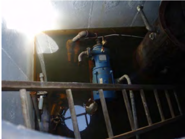
29.) Trench PUM Vent House Interior; Stoddard Odor
