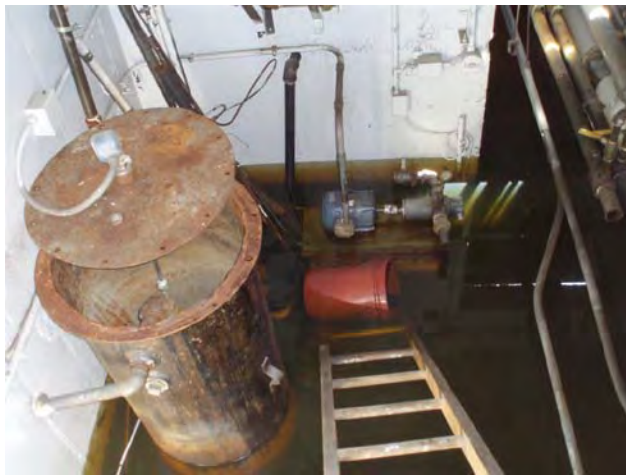
30.) Trench PUM Vent House Interior; Stoddard Odor
