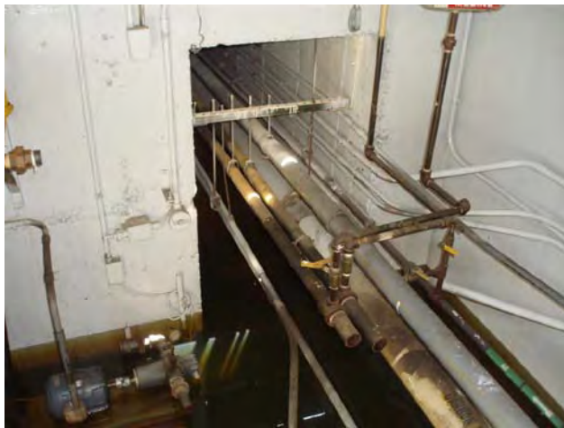
26.) Trench PUM Vent House Interior; Stoddard Odor
