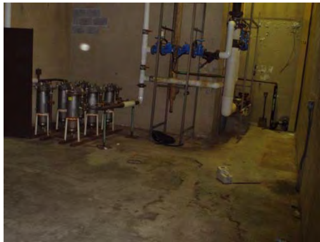
60.) Open Space A Filter Room
