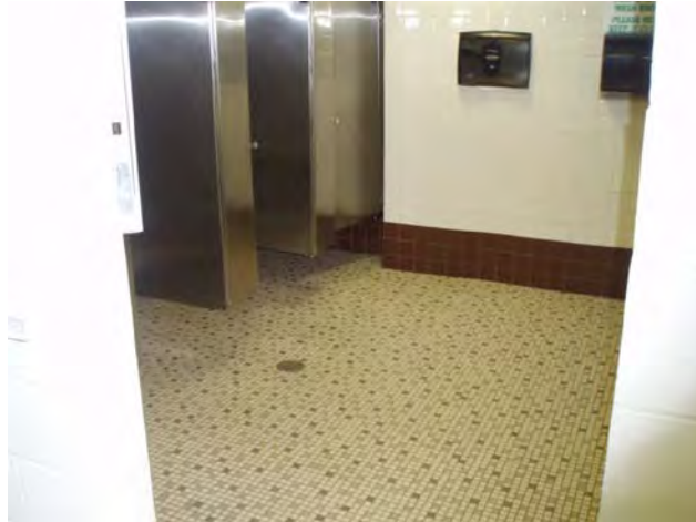
51.) Women's Bathroom Drain
