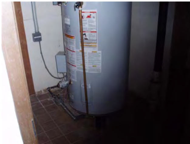
72.) Hot Water Heater Closet
