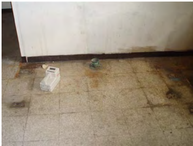
34.) Interior Rooms, Open Office C; Sanitary Drain
