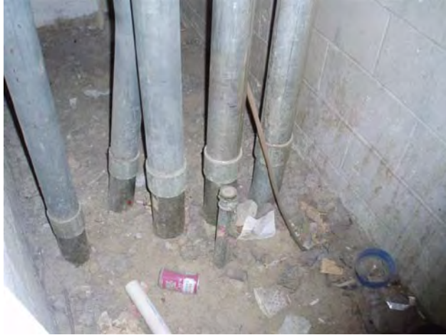
67.) Void Space Near Generators
