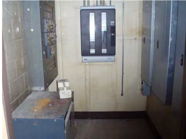
45.) Interior Open Office C Elec. Room
