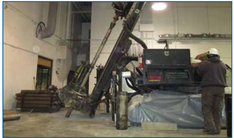
Drilling was performed inside Building 1 to further evaluate the source of contaminants beneath the building.
