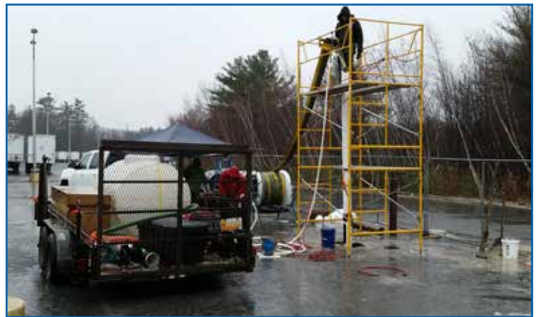
Liners were installed in bore holes to obtain groundwater samples at multiple levels.
