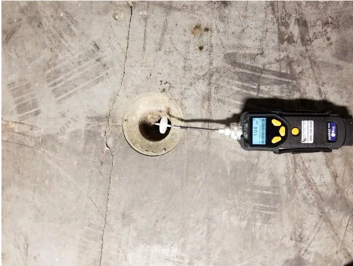
Hole in Floor_SE Corner_2
