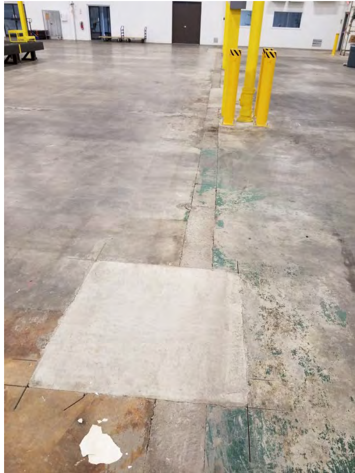
Gaps in Floor_Fisrt floor Building 1_3
