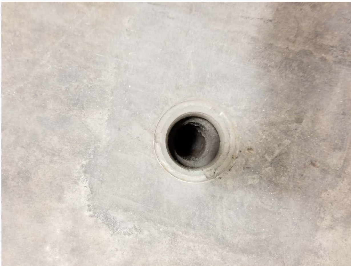
Floor Drain near IA-7_2
