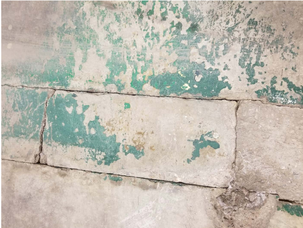
Gaps in Floor_Fisrt floor Building 1_6
