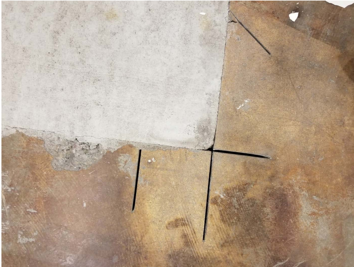
Gaps in Floor_Fisrt floor Building 1_4
