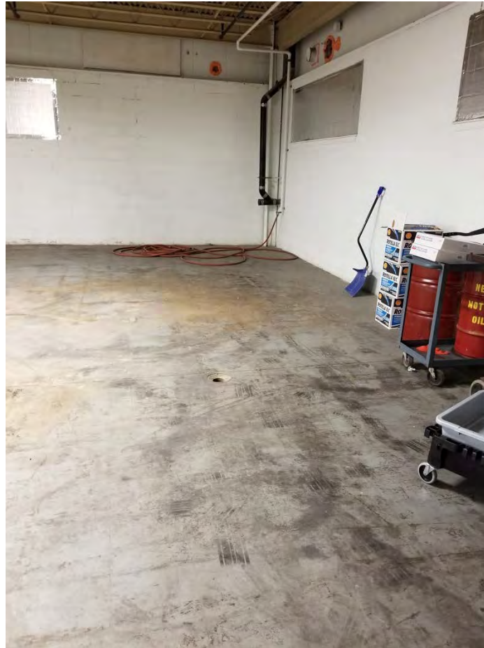
Hole in Floor_SE Corner_1
