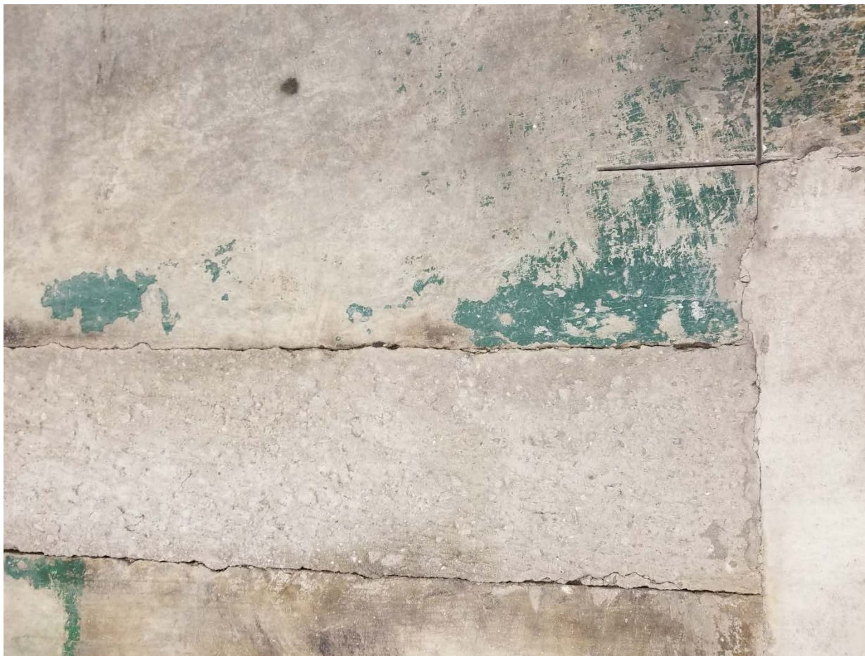
Gaps in Floor_Fisrt floor Building 1_5
