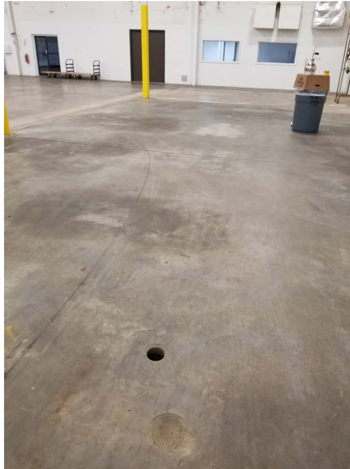
Floor Drain near IA-7_1
