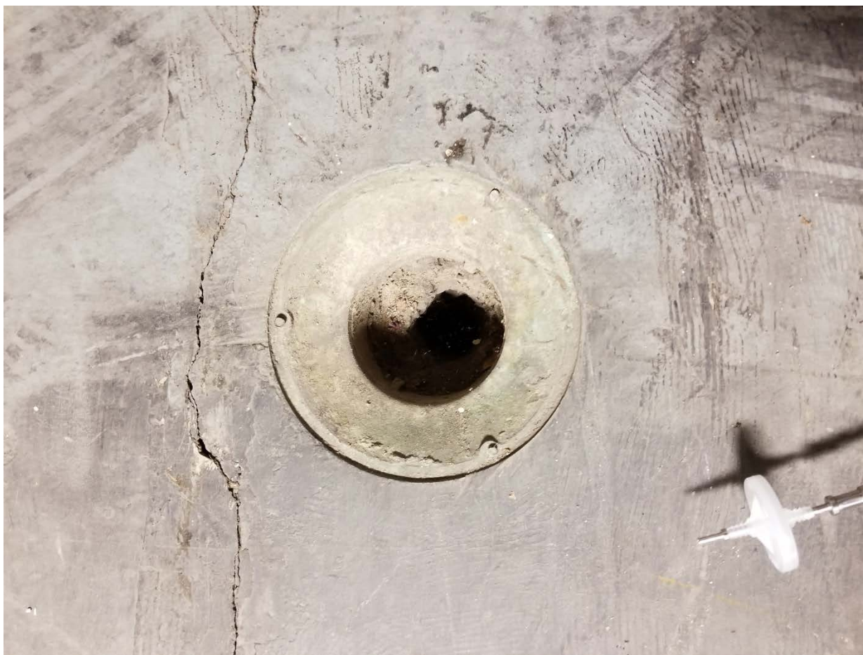
Hole in Floor_SE Corner_3
