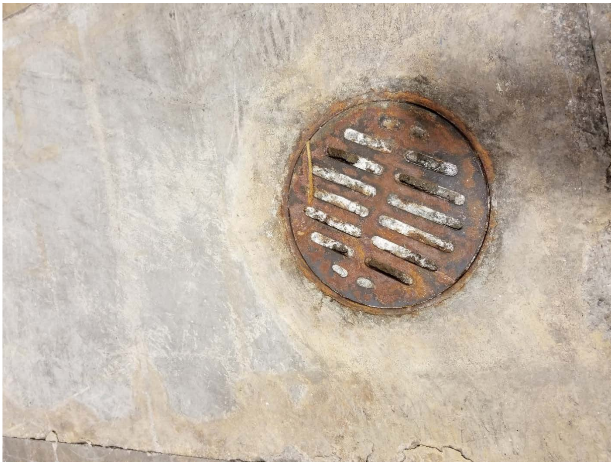
old clogged floor drain by loading docks_2
