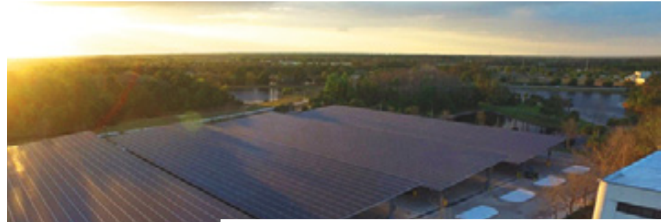
Solar Carport in Orlando, Florida.
